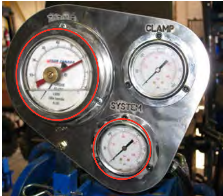
ILLUSTRATION 3.B.11: TORQUE & SYSTEM PRESSURE GAUGES ON GAUGE PANEL
