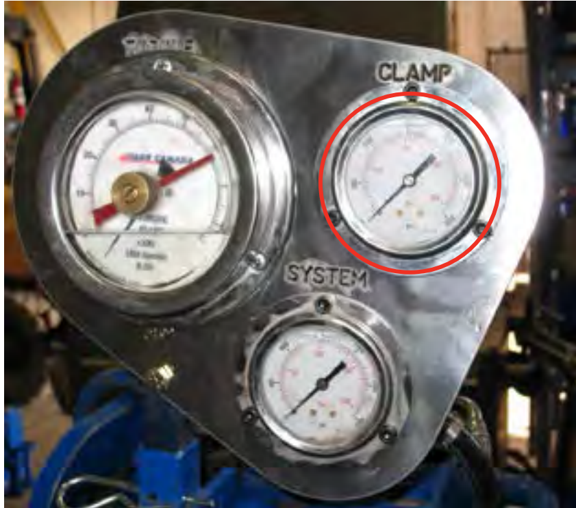
ILLUSTRATION 3.B.4: CLAMP PRESSURE GAUGE ON GAUGE PANEL
