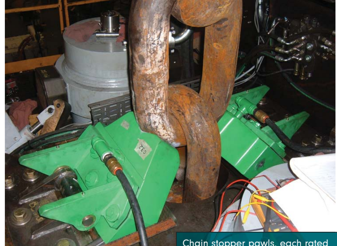
Chain stopper pawls, each rated at 1 million pound capacity
